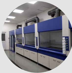
Laboratory Fume Hood
